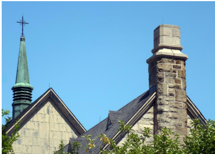
Figure 2. A chimney used by Chimney Swifts for nesting in Quebec city (photo: C. Maurice).
