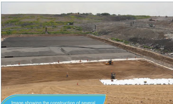
Image showing the construction of several layers of the engineered landfill liner
